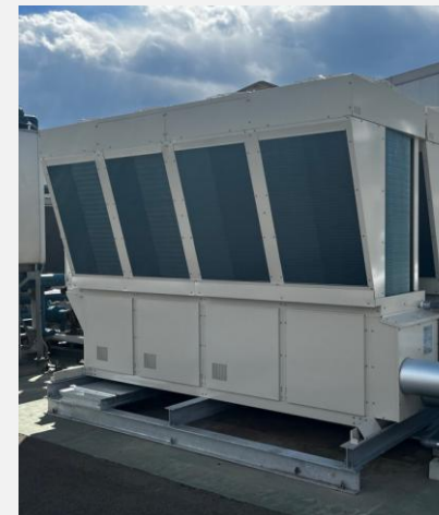
Air-cooled heat pump chiller
